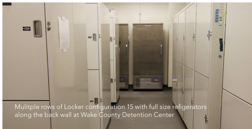
Pass-Thru Evidence Lockers at Wake County Detention Center Full size rear doors for evidence retrieval
